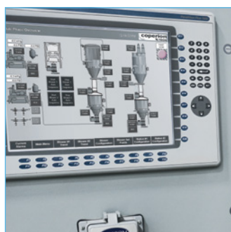
Custom PLC controls
