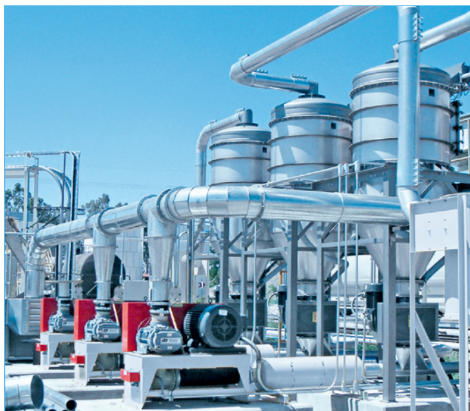
Multi ingredient silo unloading
